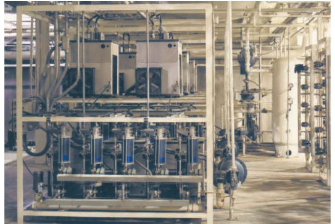
Vacuum racks with instrumentation and valving are assembled for a McGill autoclave installation.
