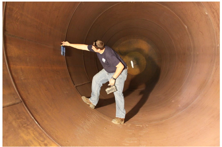
The integrity of welds done in our repairs are checked with radiographic testing.
